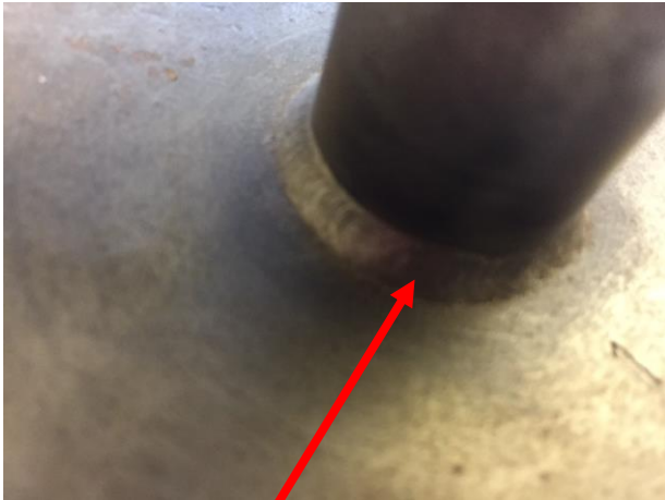
Boiler tube weld
