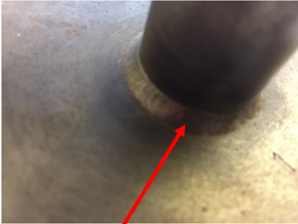
Boiler tube weld
